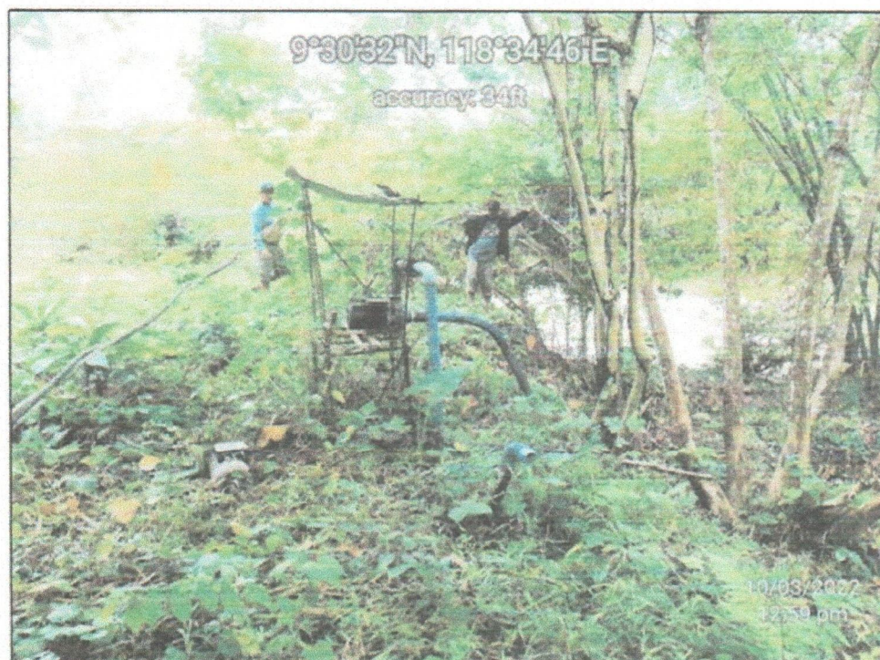
Photo 2. Water pump along the Isaub River
