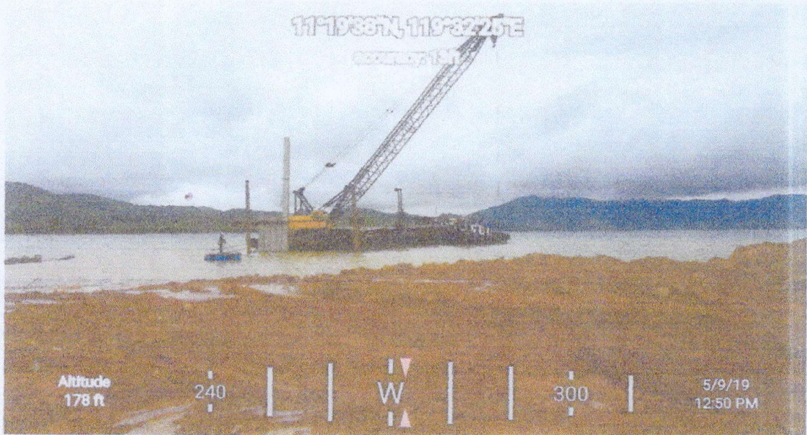
Photo No. 7: Picture of the Pile Foundation Installation project of HG-III Construction and Dev't Corp.
