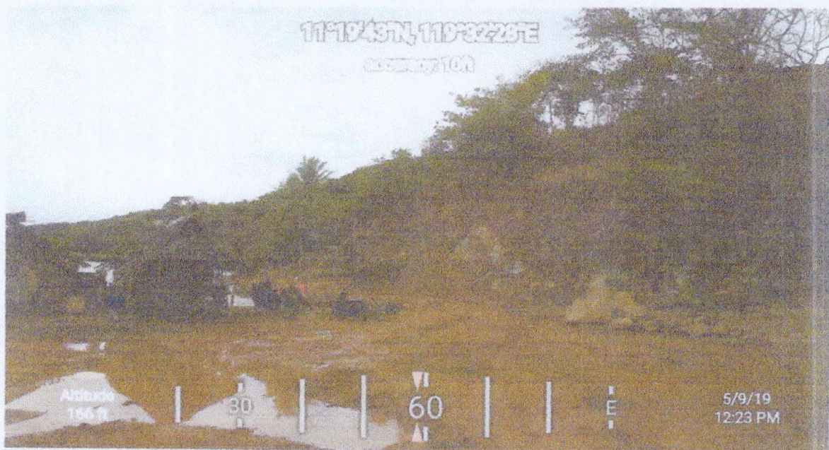
Photo No. 4: Picture of the adjacent hill where the filling materials used for the Pier Construction are extracted.
