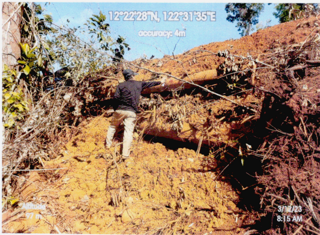
Uprooted trees dumped and filled with soil beside the perimeter access road
