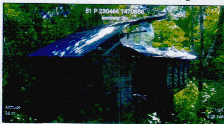
Bunkhouse damaged by typhoons
